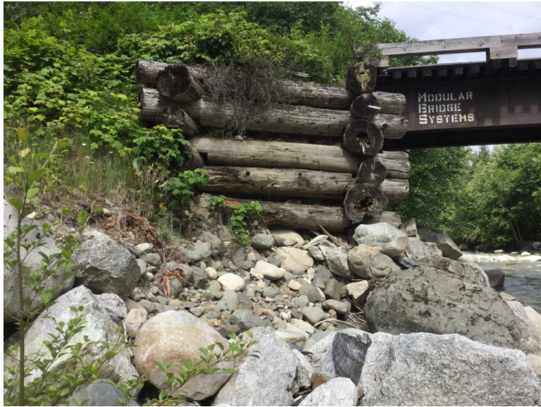
Upstream left bank scour
